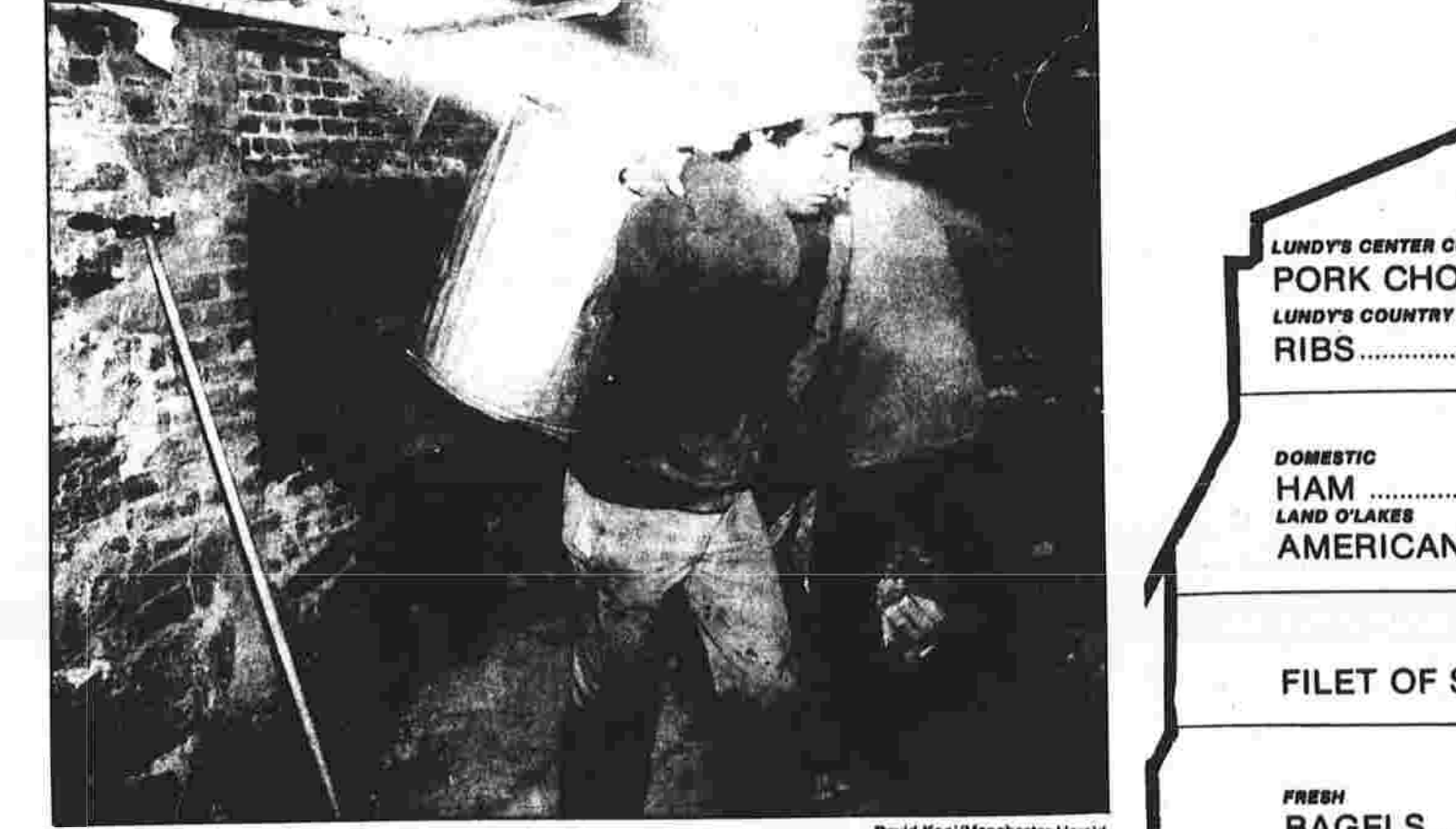
DAVID KOOL/MANCHESTER HERALD PRELIMINARY HARD WORK — John Parla of Manchester makes one of hundreds of trips through the basement of Cheney Hall last week carrying out garbage cans full of trash. Parla is supervising preliminary stages of interior renovation to the hall being done
